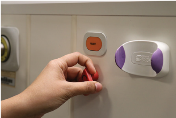
Figure 20.3 Activate the emergency button.
